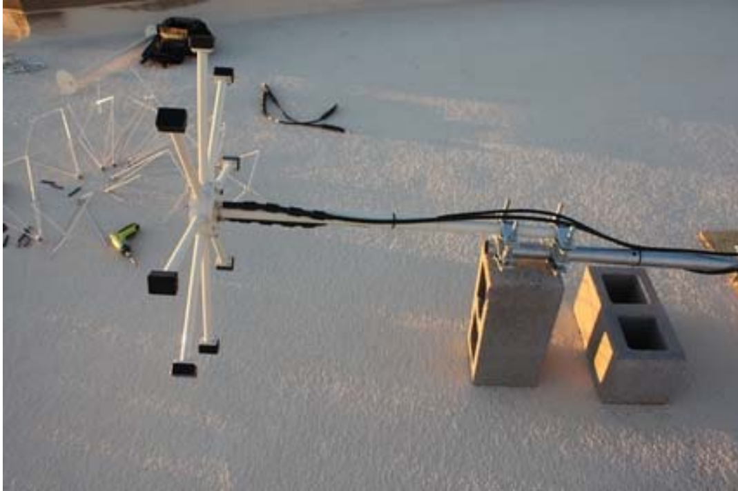
Figure 6: VHF antenna frame mounted on mast
